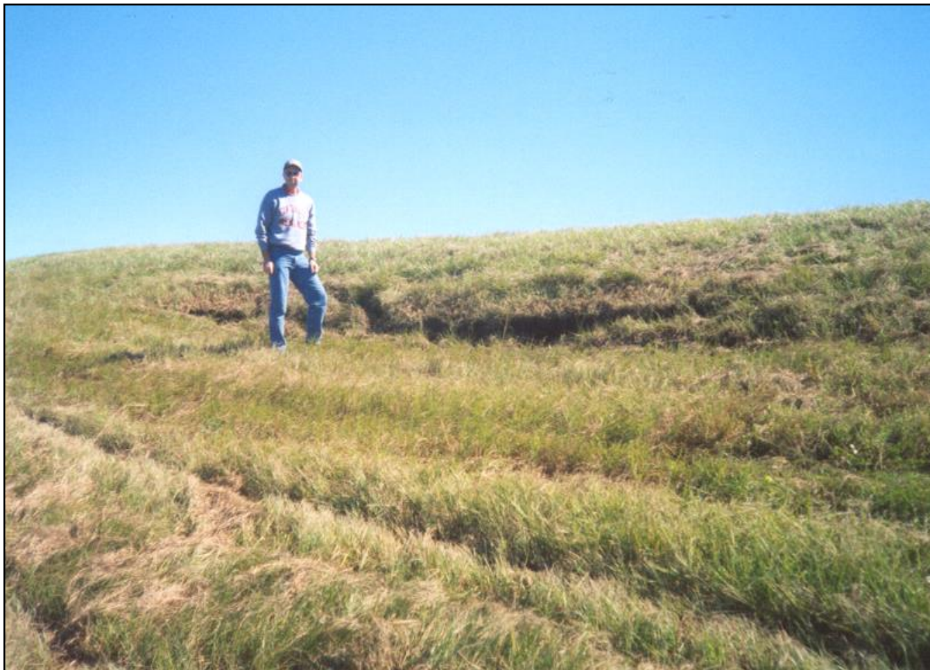
Typical final cover localized subsidence
